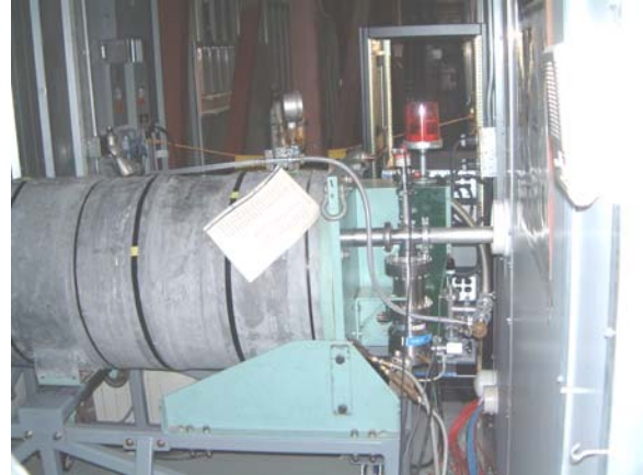
VG installed by Bldg 33 Cleanroom
