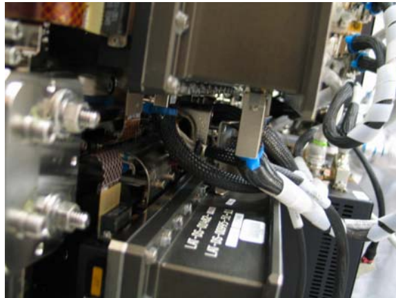
Limited access between DAQ Boxes
