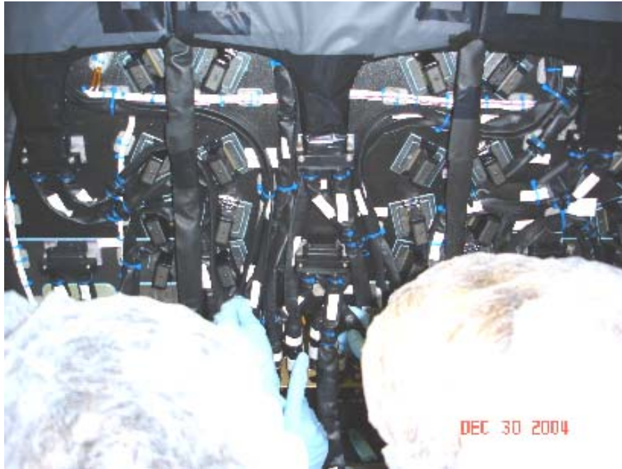
Fiber cable routing on the +Y side
